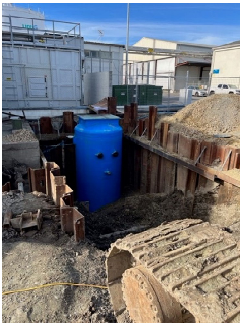
Dawson St pump station wet well.
