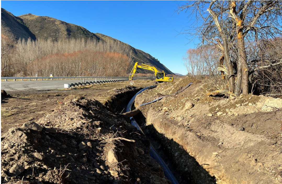
Te Ana Wai Section 2 pipeline: looking towards Rocky Gully River Crossing, going under the existing Downlands trunkmain.
