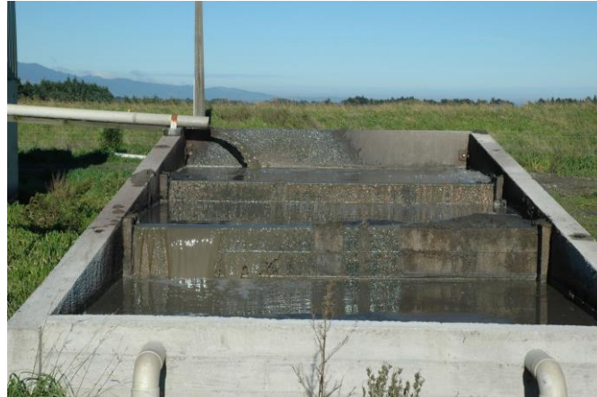
Photo 2: Example of a 'weeping' wall to collect heavy materials
