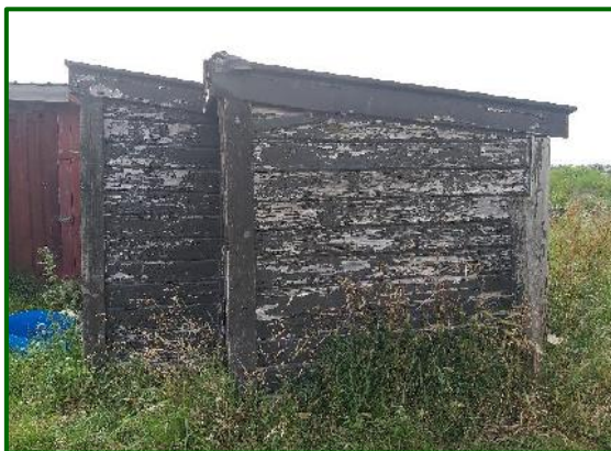
Photos 7 – Animal shed showing deteriorated paint
