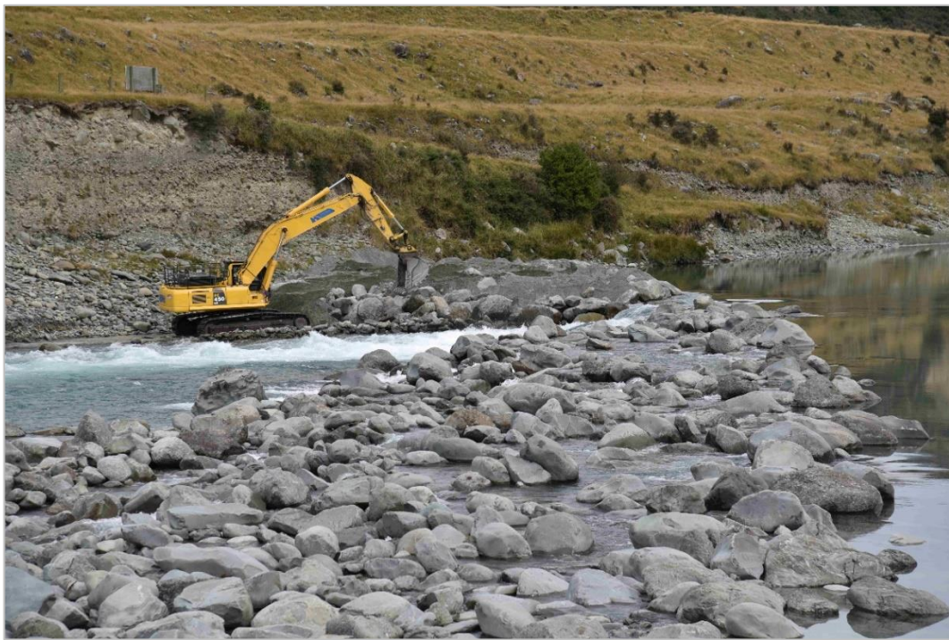
Fig 4 An excavator replacing rocks onto the right abutment of the rock weir.
