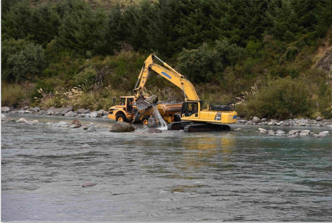
Fig 5 Recovering large rocks downstream of the rock weir to be re-placed on the weir.
