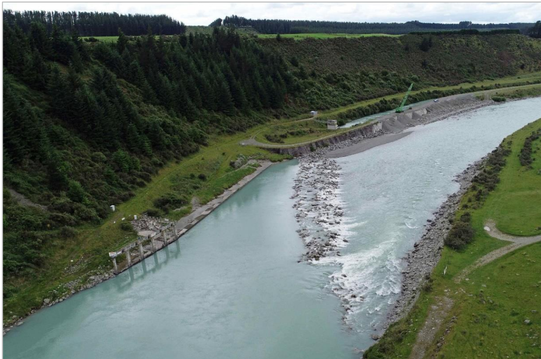
Fig 1: Aerial view looking downstream of the Scheme's intake at Klondyke. The intake is on the left bank under the six concrete pillars. The Scheme's canal can be seen running parallel to the river approximately 150m downstream of the intake. The rock weir is clearly visible, extending across the river with the
