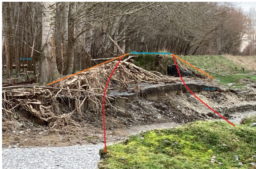
Figure 2: Section of washed out stopbank. The longitudinal crest followed the red lines, and the stopbank profile is shown by orange and blue.
