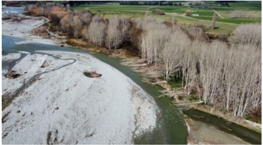
Figure 1: Aerial image of completed layering where poplars are partly cut and pushed over to stabilise an erosion site.
