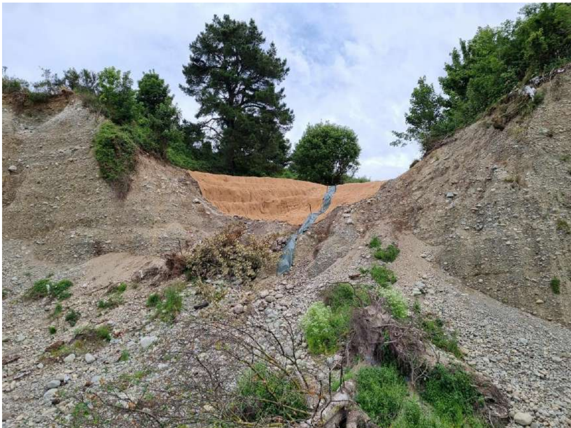
Photograph 4: View looking west from Rangitata River Bed towards gully following interim remedial works. BioCoir coconut matting and Flexiflume piping visible. (December 2022)
