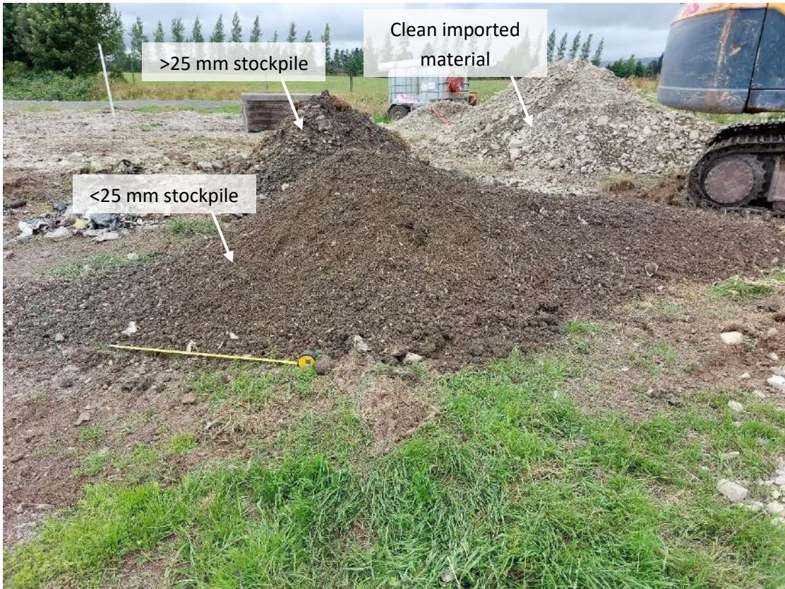
Photograph 18: TP103 <25 mm screened stockpile in foreground. >25 mm screened stockpile can be seen behind.
