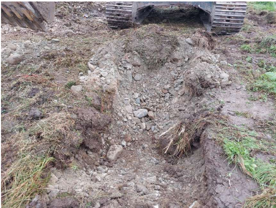
Photograph 22: 'Cover' material observed in TP104.
