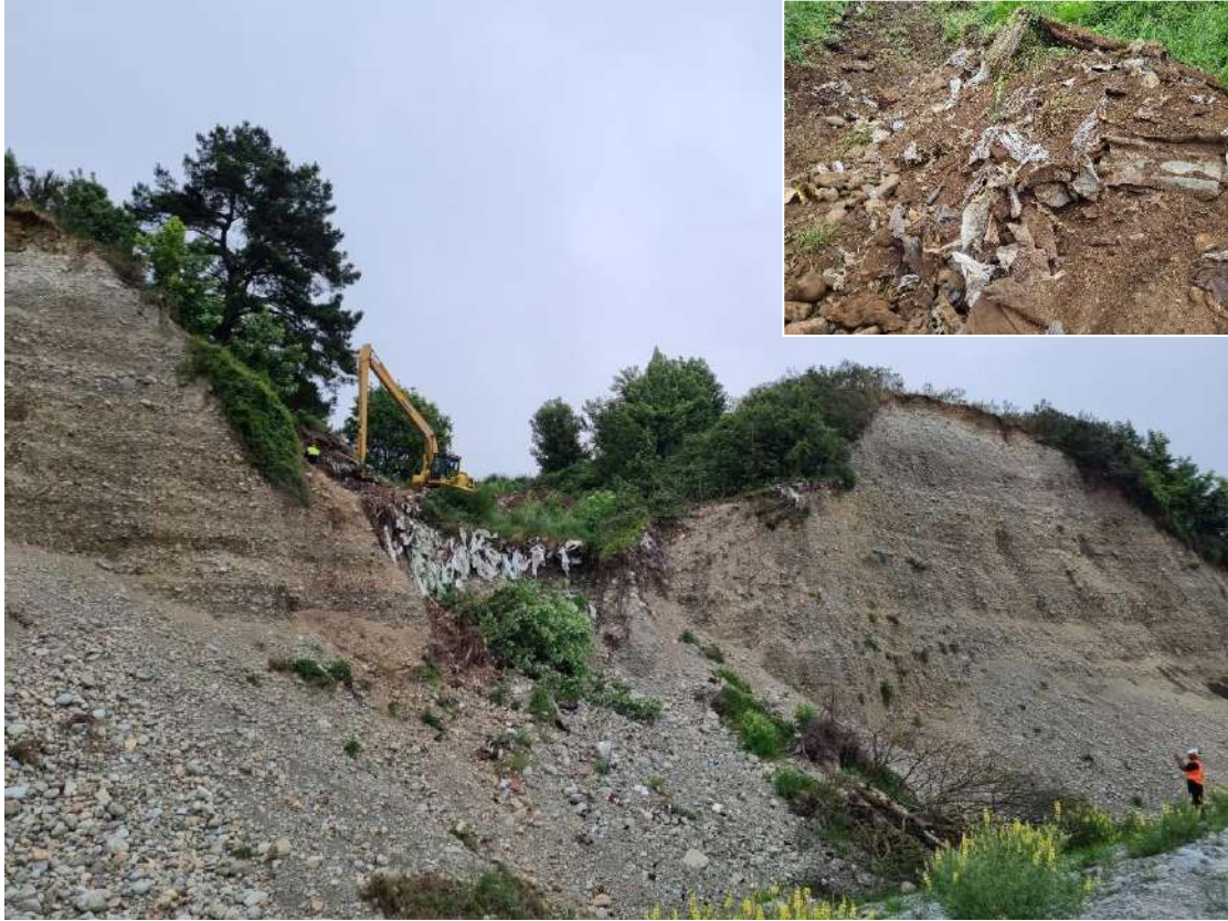
Photograph 3: View looking north west from Rangitata River Bed inspection towards gully during interim remedial works. Waste materials can be seen to have fallen into the toe of the terrace. Inset shows waste materials encountered. (December 2022)
