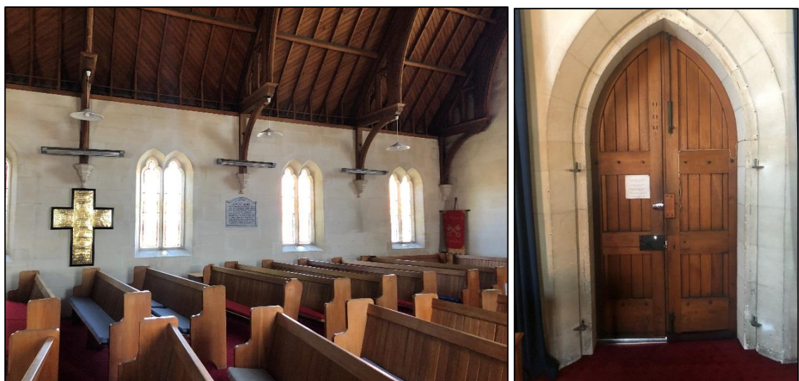
Left: South wall of nave. Right: Door to church from entry porch. Source: DPA Architects, January 2020.
