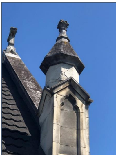
Weathering and soiling of limestone to pinnacle. Source: DPA Architects, January 2020.
