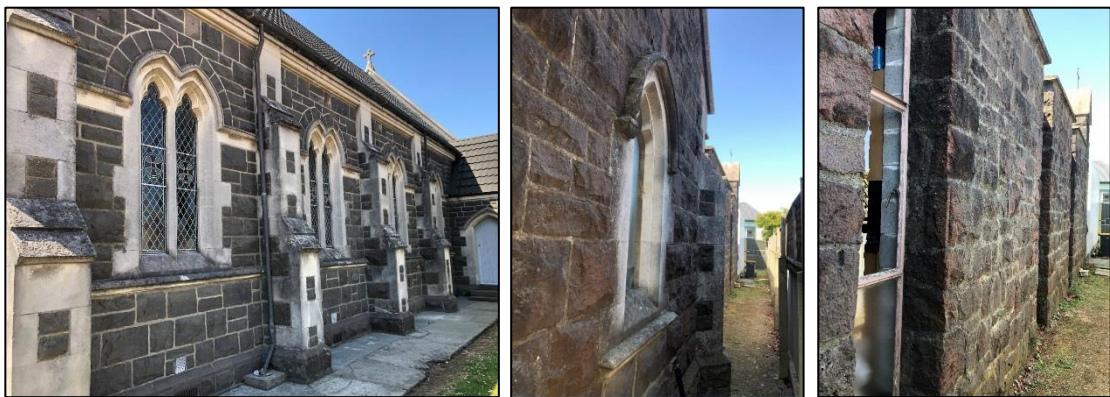
Left and Centre: Soiling of limestone and moss growth. Right: Cracked and missing putty to window joinery and lichen growth to stone. Source: DPA Architects, January 2020.
