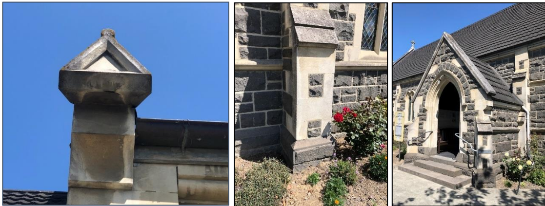
Left: soiling of limestone. Centre: Possible horizontal displacement to stone base of buttress. Right: Handrails and plastic downpipe to entry porch. Source: DPA Architects, January 2020.
