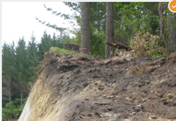
Example of good road-line salvage with a sufficient number of trees removed providing adequate width road formation.
