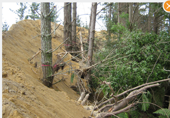
Example of poor road-line salvage where adequate allowance has not been made for road formation and fill has been run into standing trees.
