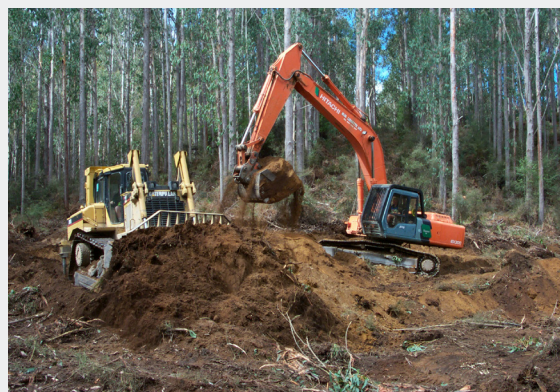
Excavator and bull dozer clearing stumps and stripping prior to bulk earthworks.
